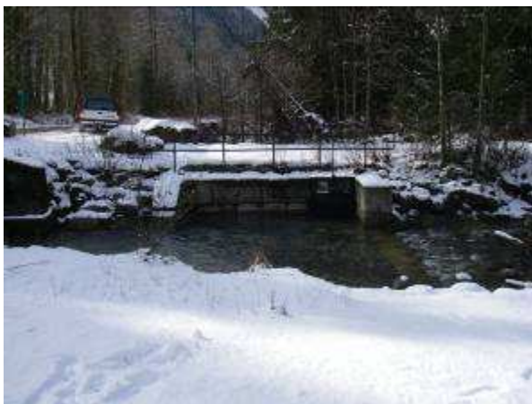
Borden Creek side channel complex intake location, still functional and stable, Chilliwack watershed.
