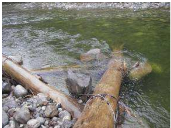
Close-up look at the LWD structures placed on Big Silver Creek, structure is showing some signs of instability and may need some attention.
