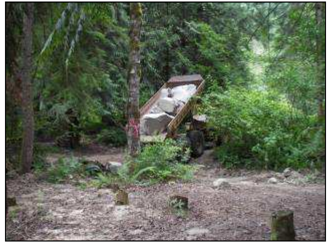
Off-loading rock; used as bank protection, or as ballast material to hold the wood structures in place.
