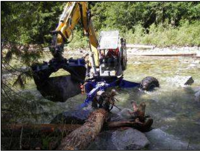
Construction of the wood habitat structures using the environmentally sensitive spyder excavator.
