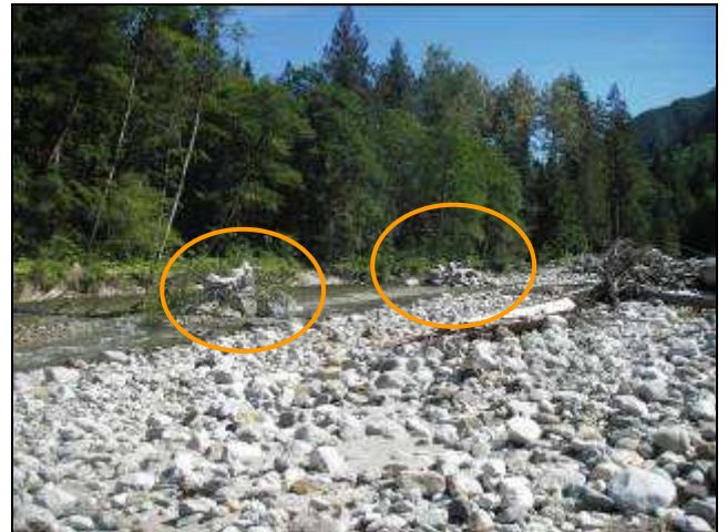
Staging material adjacent to the sites where installation of the wood structures is to take place.
