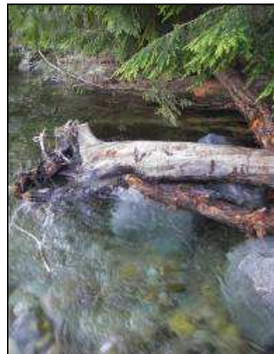
View looking from above, on a portion of the parallel wood structure.
