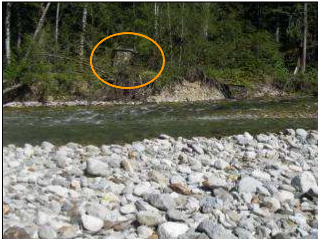
Pre-construction eroding stream bank. Note the size of a tree stump which once protected the bank.
