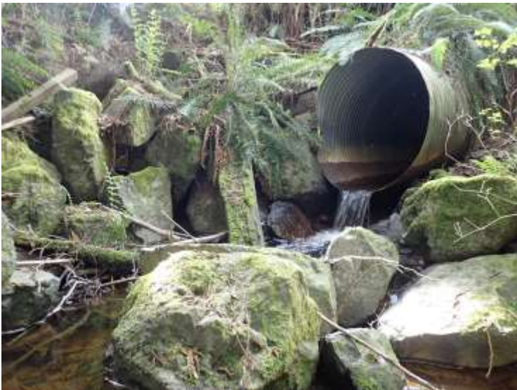
Little Anderson Creek
