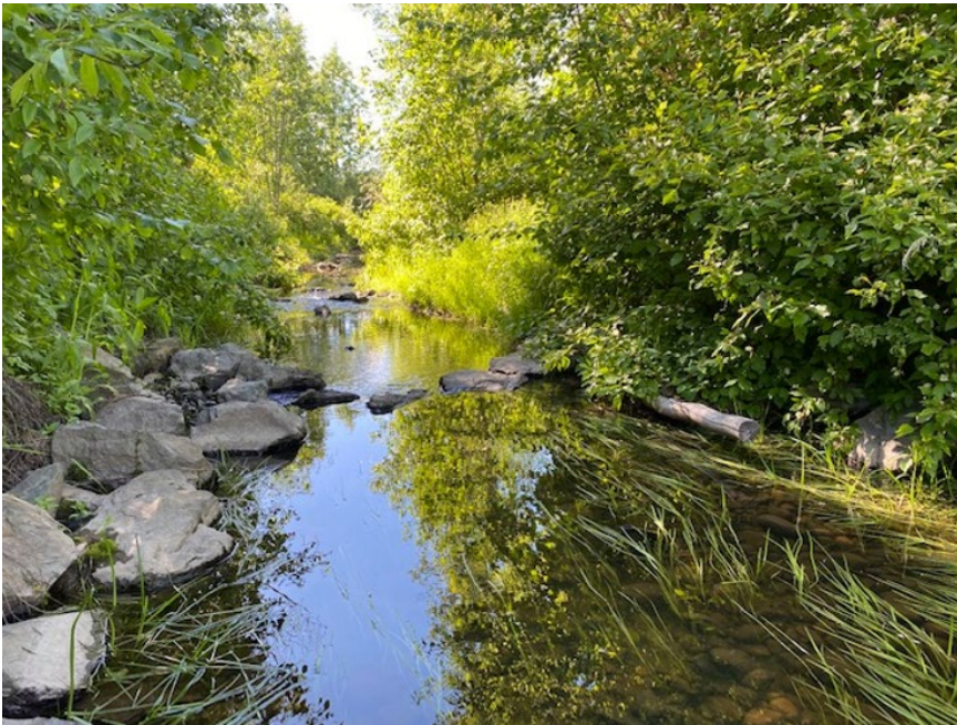
Boulder placement within a side channel restoration project (Photo Credit: Wayne Salewski)
