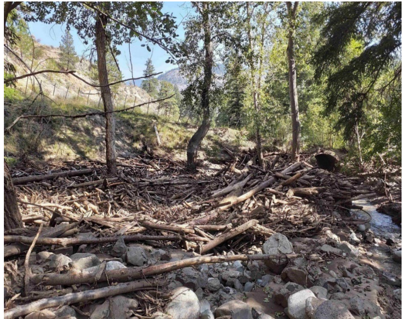
Debris buildup upstream of culvert inlet (Photo credit: Pacific Salmon Foundation)
